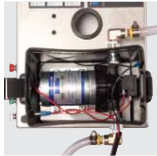
12V Booster Pump is protected in an all-weather box.
